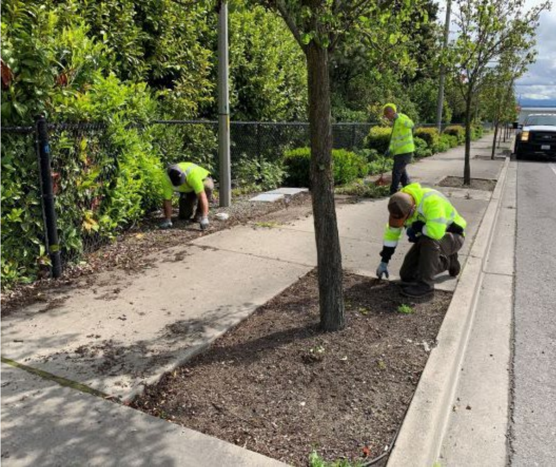
Public Works Maintenance at South 154th Street Photo courtesy SeaTac Public Works Department
